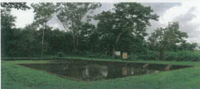
Surface Rain Water Harvesting System at colony
